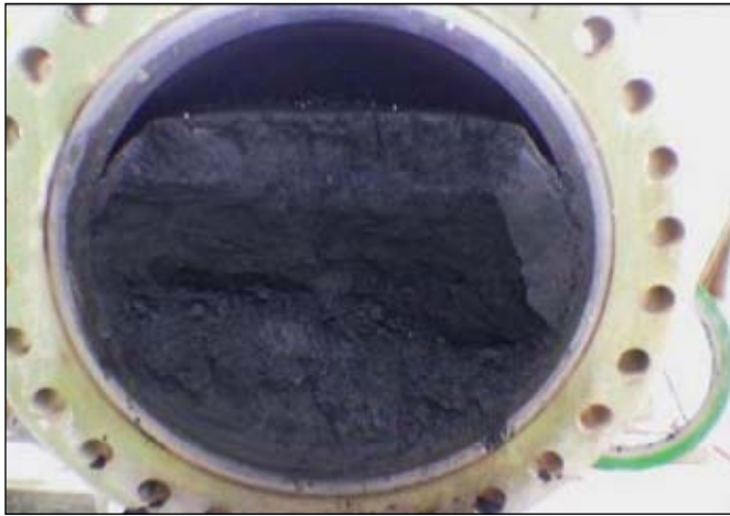
Wet tar-like black powder can collect at scraper door receivers of dry gas pipelines. This photo shows an accumulation at such a location on Saudi Aramco's gas transmission system (Fig. 1).
